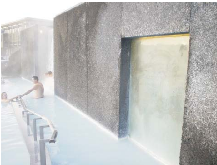
Heavy silica contamination on a glass door at the Bláa Lónið resort prior to ClearShield renovation and protection
